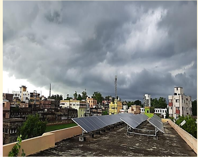
Solar Panels installed at the College
